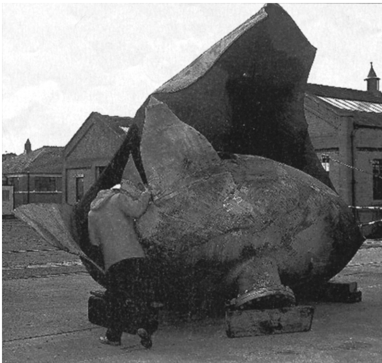
FIGURE 28-1 The result of an absorber failure. From reference 18. (Reprinted with the permission of Gulf Professional Publishing.)
